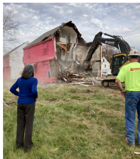
Mayor Maggard of Whitehall watches as a property in the Woodcliff complex is demolished. COCIC is managing the demolition of the entire complex.
