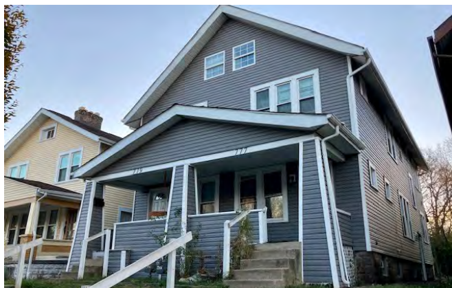
COCIC provided a low-interest loan to the court-appointed receiver that rehabbed this Driving Park duplex.
